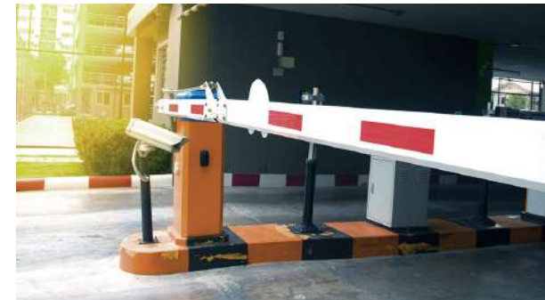
Vehicle Access Control
